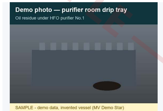
P3 RISQ 13 / 13.29 - Demo photo - oil residue in purifier drip tray (27 Sep 2026)
