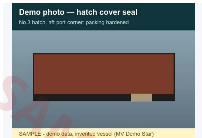
P1 RISQ 9A / 9.9 - Demo photo - No.3 hatch cover rubber packing, aft port corner (25 Sep 2026)
